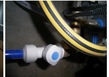
water heater supply valve
